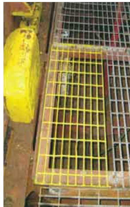
▲ THE GRATES WERE ORIGINALLY DESIGNED SO THAT THEY WOULD ONLY BE SECURE IF THEY WERE PLACED CORRECTLY, HOWEVER, THE DESIGN MADE IT EASY FOR THE GRATE TO BE INADVERTENTLY REPLACED BACK-TO-FRONT.
