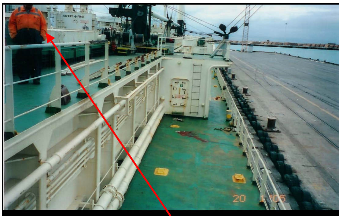
PHOTOGRAPH OF HATCH DECK (MAN IN ORANGE) AND IMPACT AREA ON MAIN DECK BELOW.
