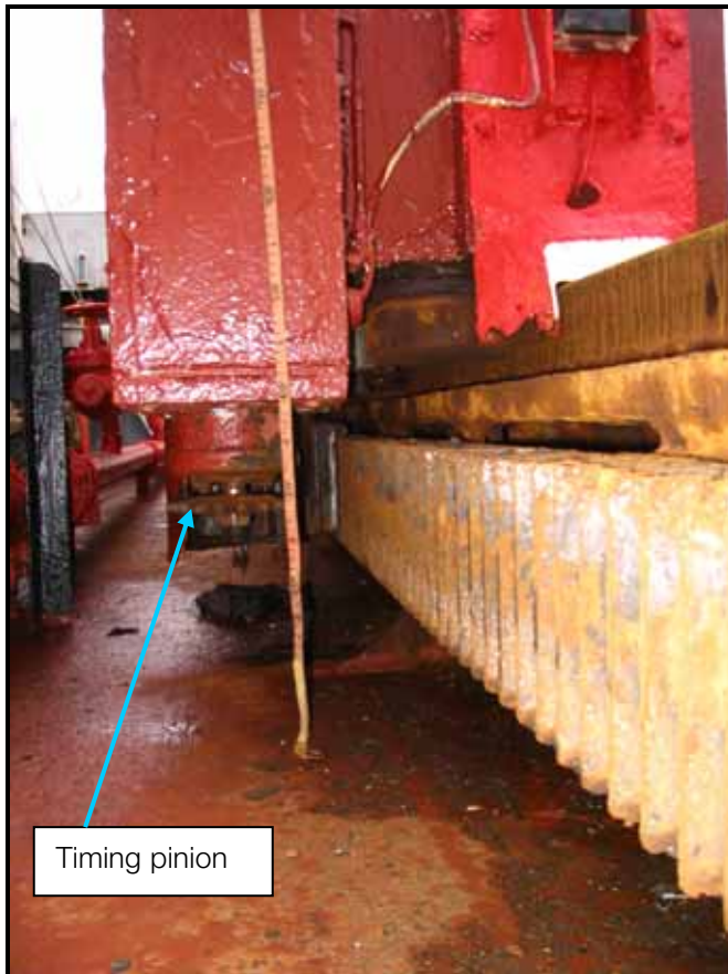
Photograph 5 Unguarded pinion viewed from aft
