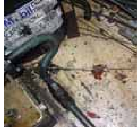
BROKEN FLEXIBLE PULL WIRE REPAIRED WITH A KNOT.
